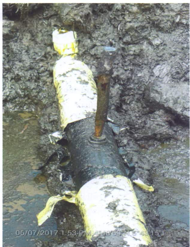
LEAK POINT PEGGED
